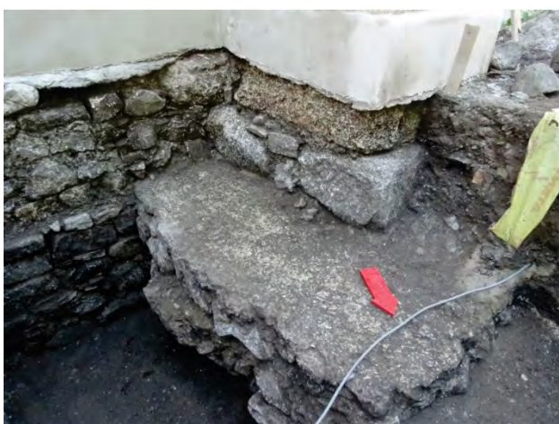
Figura 27. Fundația celui mai de vest contrafort perpendicular nordic / The foundation of the westernmost northern perpendicular buttress.
