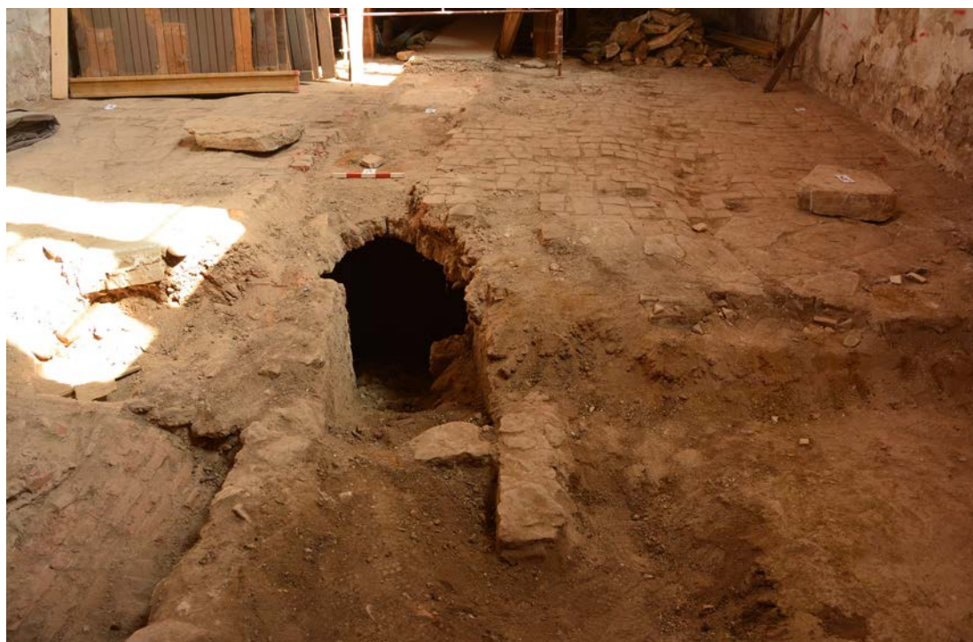
Fig. 1. Collapsed vault in the sanctuary of the Calvinist Church in Huedin (image from the MNIT Archive).
