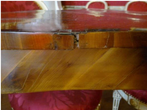
9. Detail; reattachment on the plywood layer level with synthetic adhesive with fluidity in a warm environment
