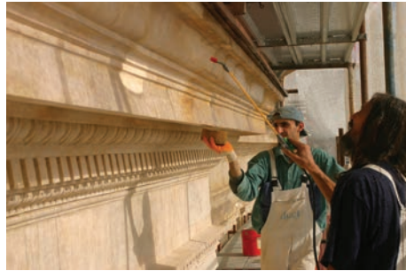
Fig. 24 - Tratamentele protective al suprafetelor de calcar cu o substanta hidrofuga, fațada Lipscani / Protective treatment of the limestone surfaces with a water repellent product, the Lipscani facade.
