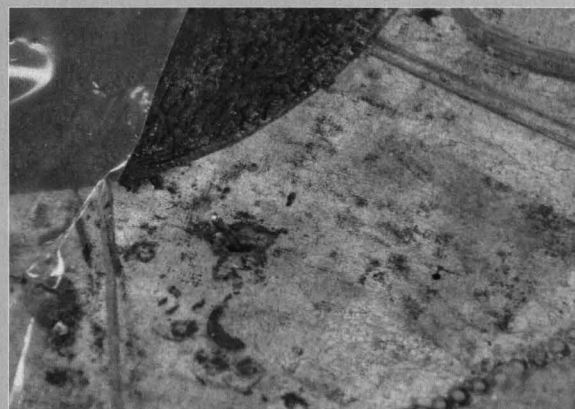
Fig. 8 - Urme de cuie. Detaliu Fig. 8 - Traces of nails. Detail
