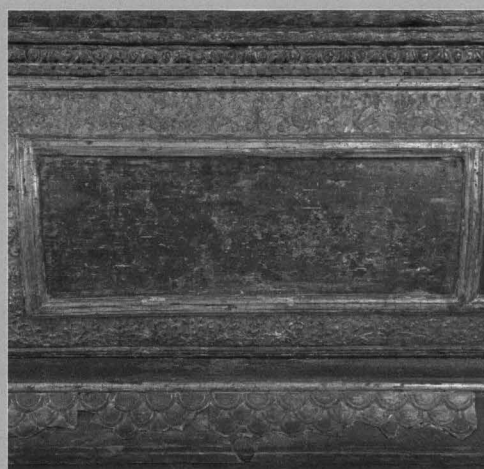
Detaliu degradare casetă fronton central Detail on degradation of central gable box
