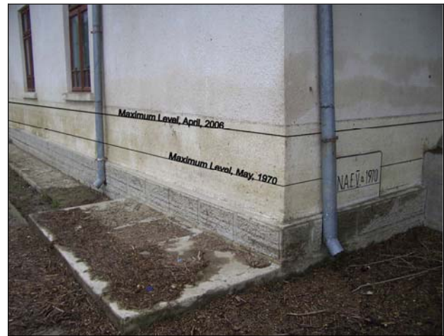
Figure 3. Bechet Harbour Building, with the marks of 1970 and 2006 floods (photo by Boengiu S.).
