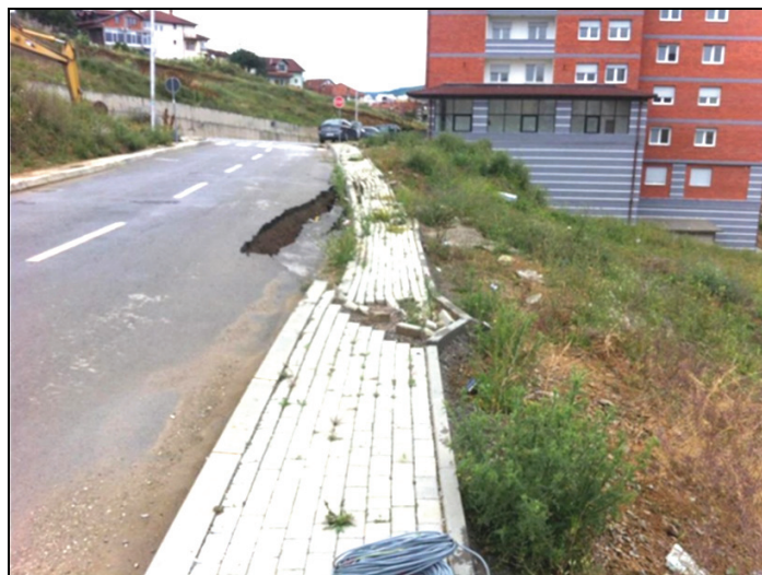
Photo 1. Landslide spot evidenced by road damages (original).
