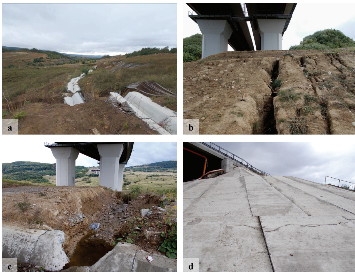
Figure 3. Photographs of the highway construction works (original, September 2017). a) Broken collecting channel on the cutting slope (Bucium Hill). b) Gullies at the pilots down the eastern head of the Aciliu Viaduct. c) Broken collecting channel and the subsequent gully at the western head of the Aciliu Viaduct. e) Cracked and dislocated concrete slabs at the western head abutment.
