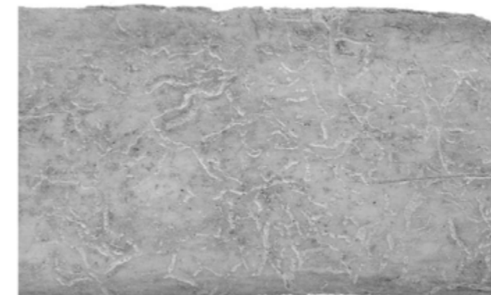
Pic. 19. plant-root erosion on a rib, Cx211
