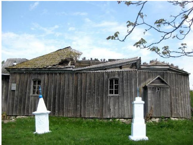
Photo 1. The demolished wooden church “Saint Archangel Michael”, Hiliuți, Râșcani
