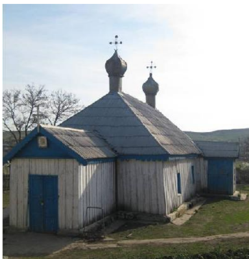
Photo7. The destroyed foundation and wood of the church
