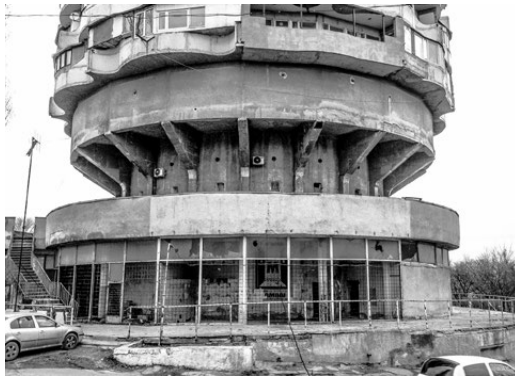
Photograph 6: Current state of the building illustrated through a picture of the former commercial spaces on the ground floor. © B.A.C.U. photo department/2016.
