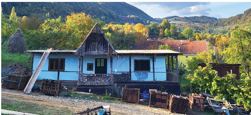
Paul Lușca and Simion's house from Cămârzana while it was demolished in 2023. Photo credit: Mihaela Grigorean.
