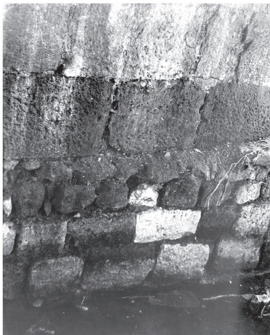
Fig. 5 - Section of the earlier fortress wall employed as a foundation for the 6 th c. fortification. Photo from the excavations of the eastern gates of Drastar.
