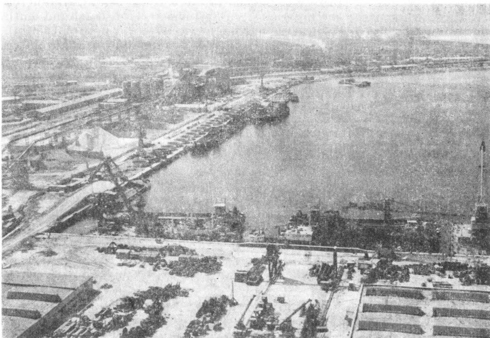
Fig. 4. — Partial view of the new port Constanța South — Agigea in construction (photo Agerpres).
